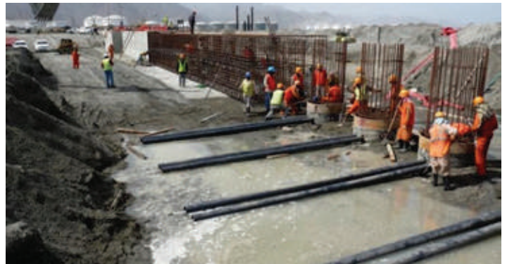
OT2 OIL TERMINAL, UAE
