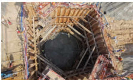
STORM WATER PUMP STATION, UAE
