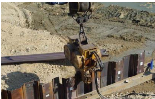
Drive the sheet piles after the drying the DPS-500 (after one day).
